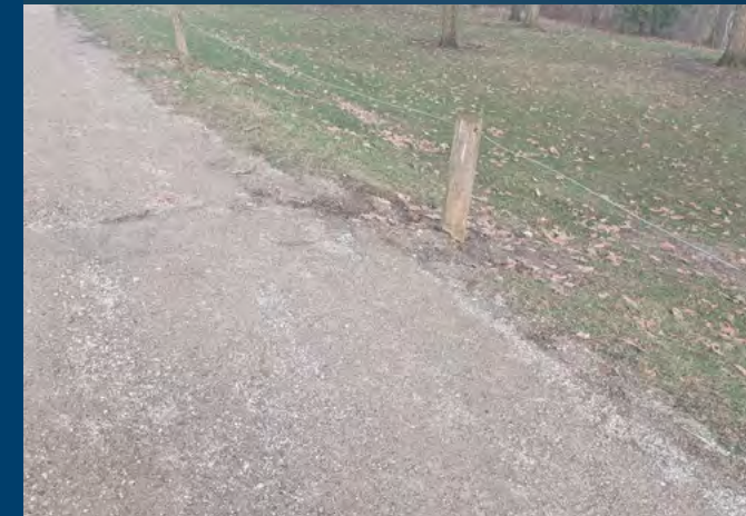
William Street shoulder erosion
